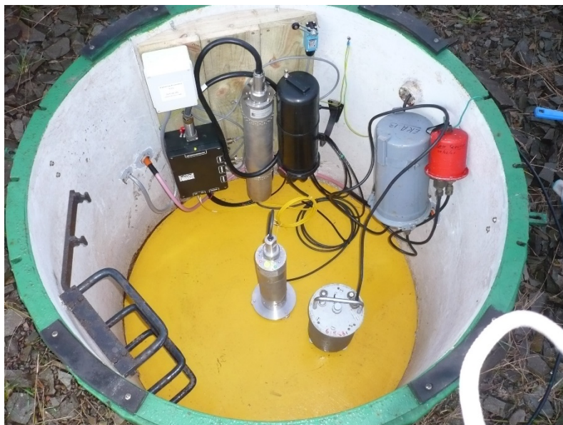
Figure 3. One of the Eskdalemuir array pits containing 3V seismometer, DM24 digitiser and acquisition system
