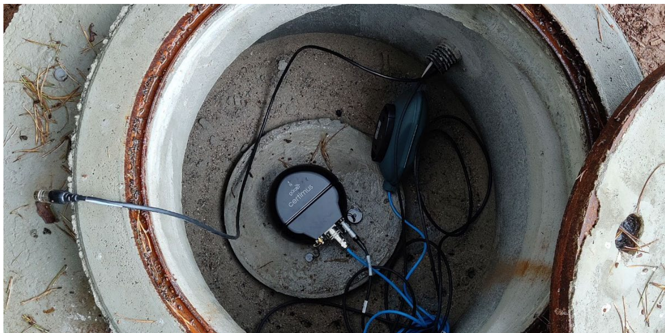
Figure 1 Installation of a Certimus seismic station forming part of the array. Image provided by Dr. Philip Hering, Goethe-University
