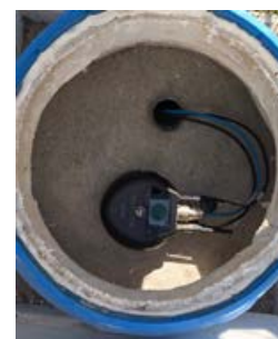
Figure 3: The Fortimus is installed in a thermally insulated vault
